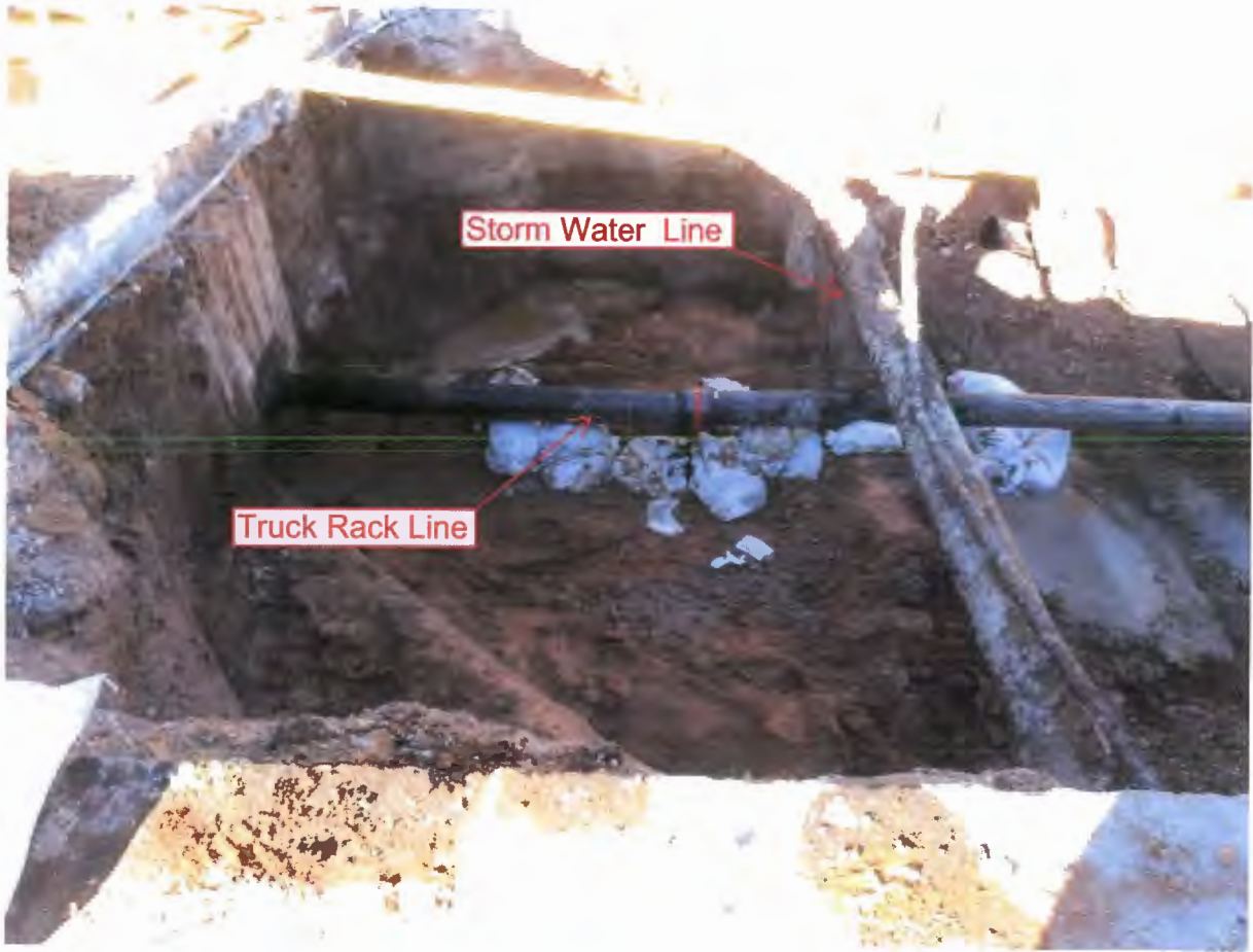
Photo of replaced sewer line near south end of excavation looking to the west.
