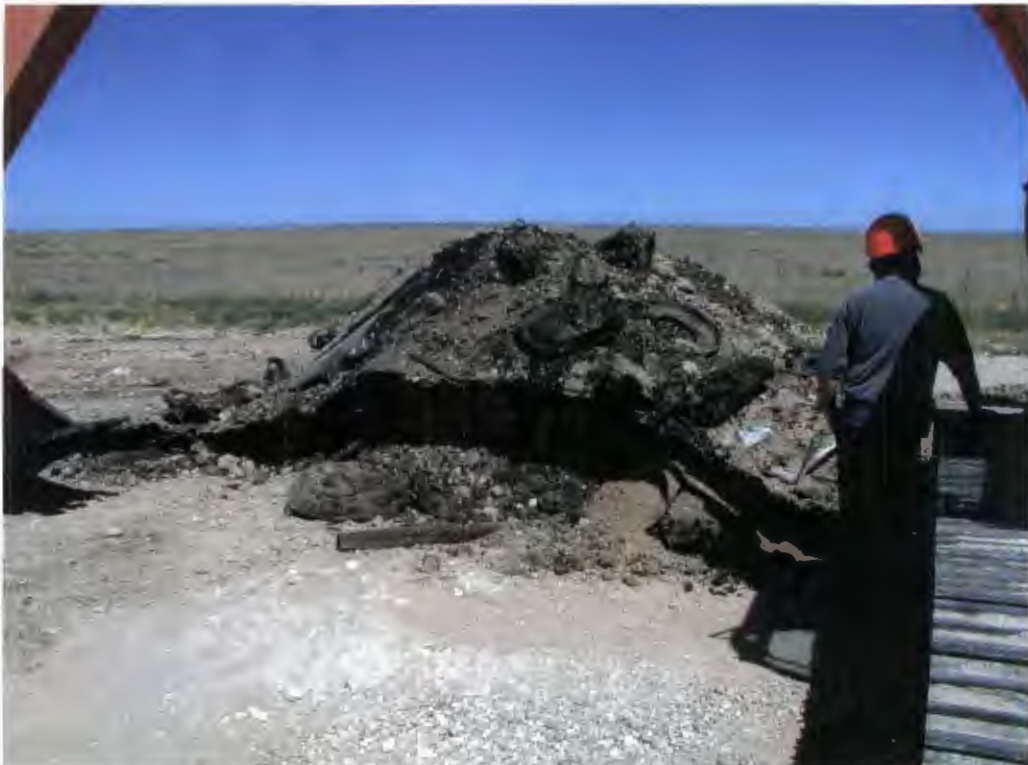
Soil and debris excavated from the east trench in the former Pit #1 area.
