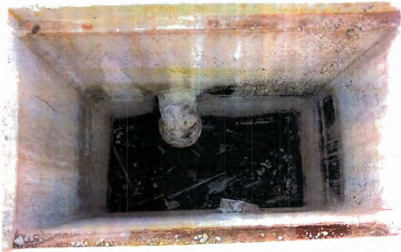
Photograph No. 4: Concrete Sump Interior (Note: The dimensions of the concrete sump are as follows; length = 4 ft, width = 2.5 ft, depth = 5 ft.)
