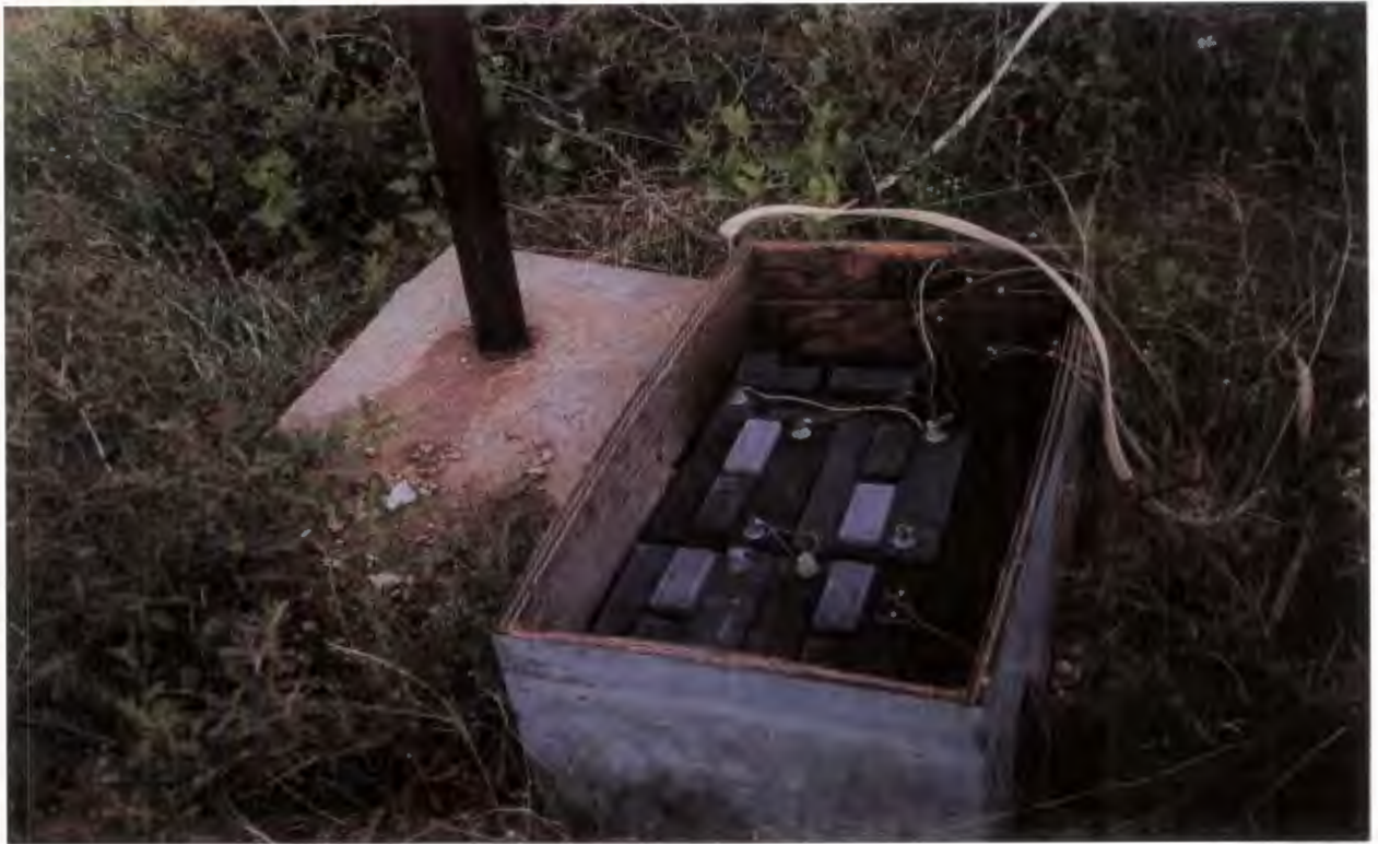
Battery Box Near the Wind Vane
